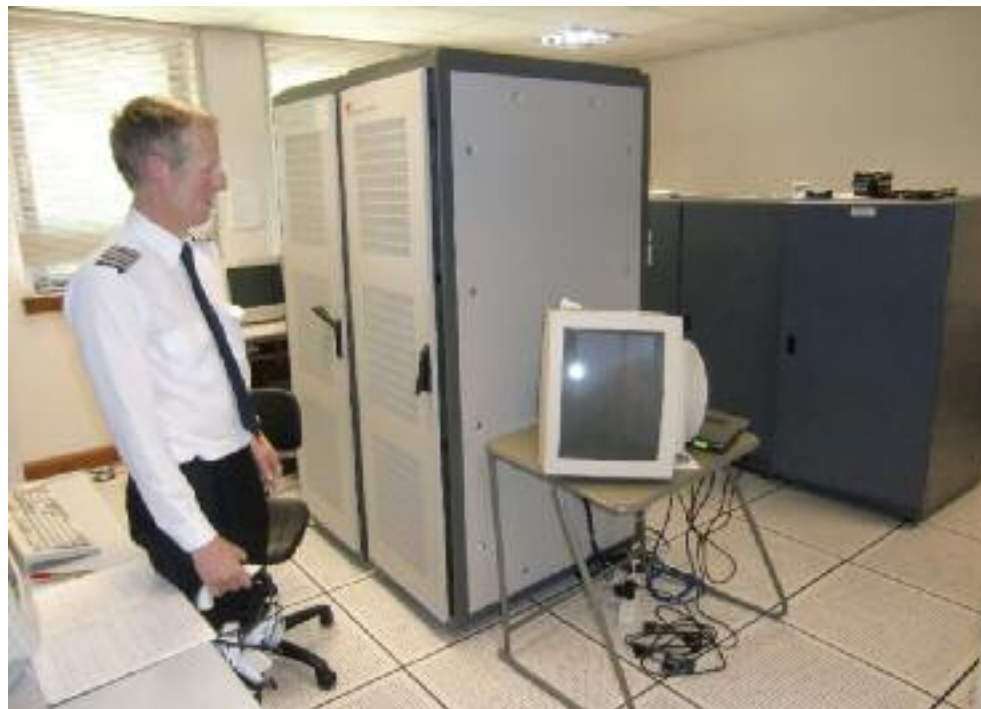
Left: computer control room – tall cabinets for movement, darker cabinets for graphics Bottom left: hydraulic pumps generate serious heat – doors and windows must be left open
